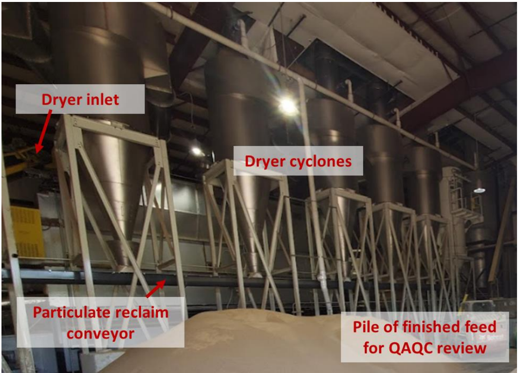
Figure 5: Photographs of as-installed equipment
